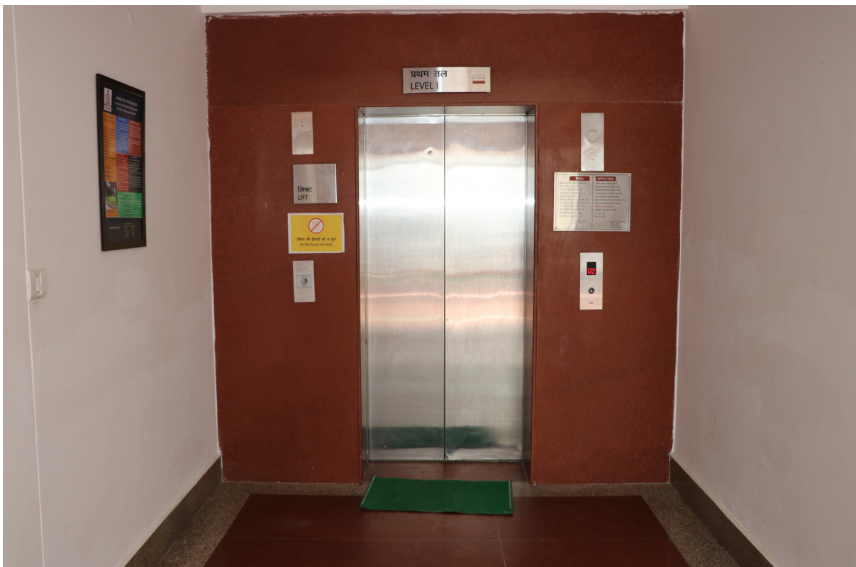
Figure 1.15: Lift for Mahanadi hostel
