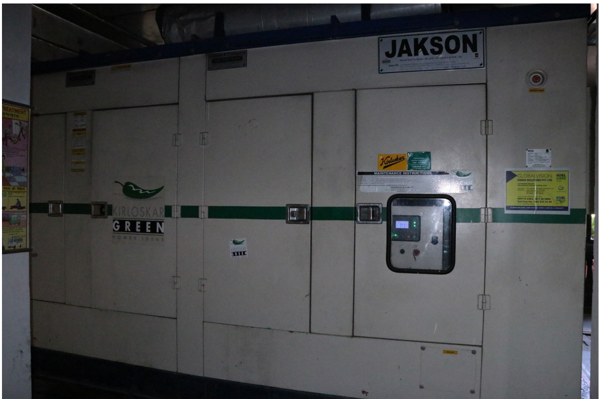
Figure 1.9: Campus electricity generator
