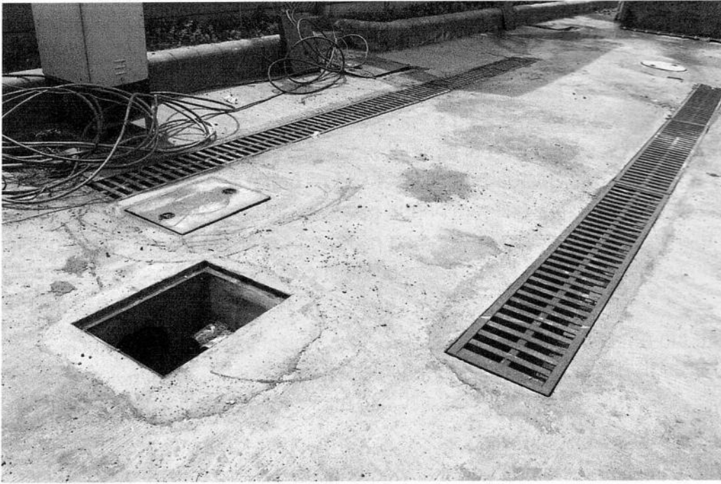
Fig 5.5 RWH by Pit method at San martin Flats, Chanakyapuri
