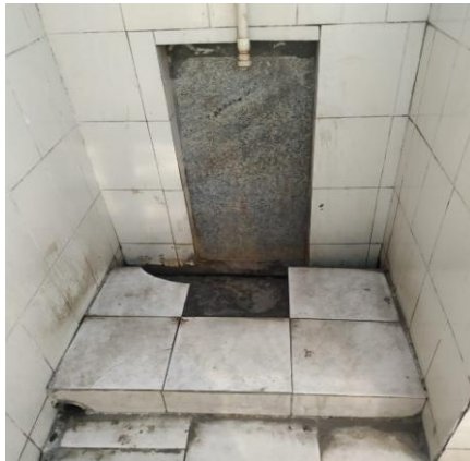
Photograph 31: Urinals connected to open drain
