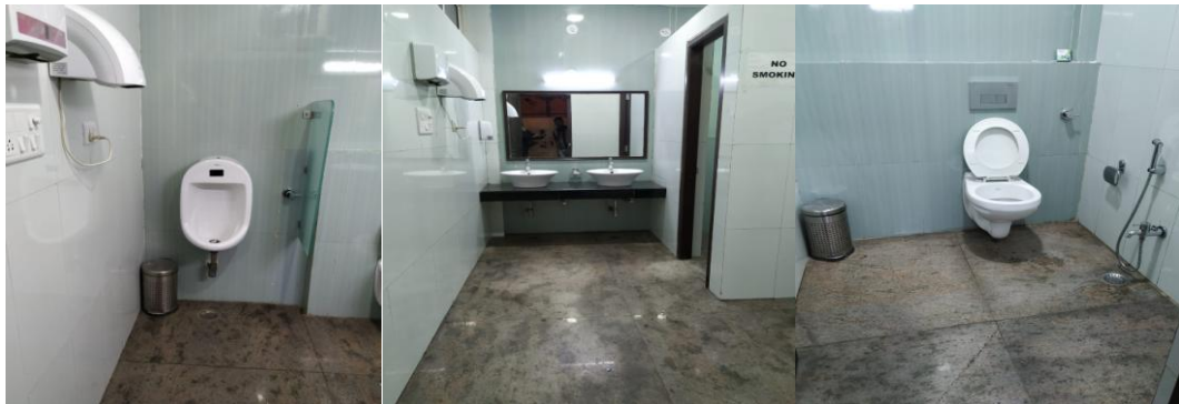
Photograph 25: New PT at Shastri Bazaar, next to P&T Colony(Internal)
