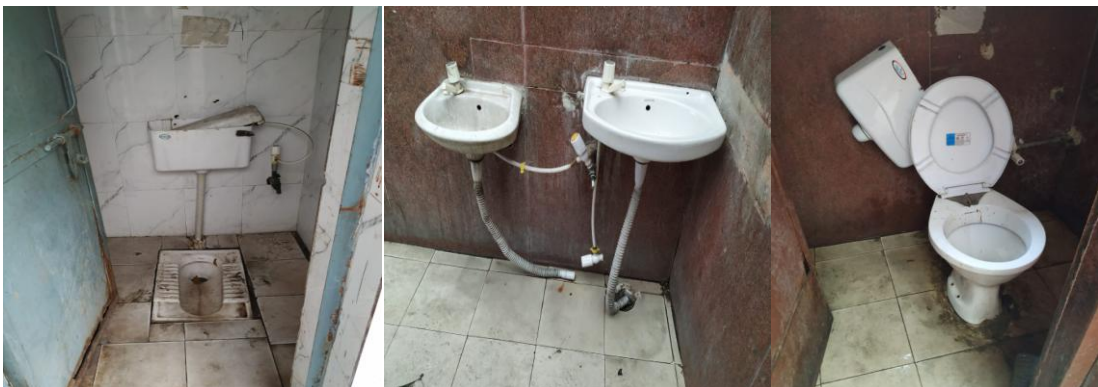
Photograph 39: Broken Fixtures at PTs
