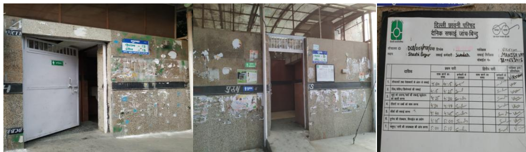
Photograph 22: Old PT at Shastri Bazaar (External)
