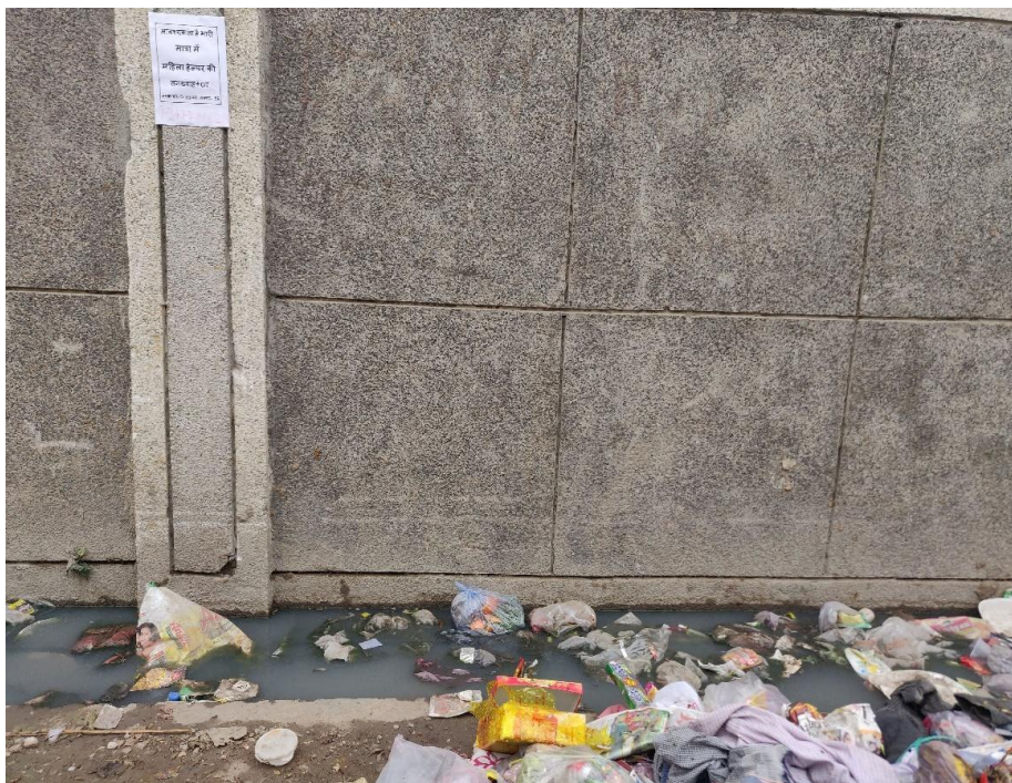
Open drains outside the PHC premises
