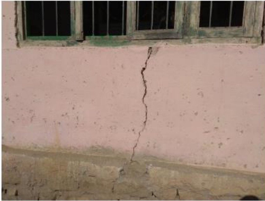
Picture 5.1 Risk Description: Cracks in the school building during earthquake
