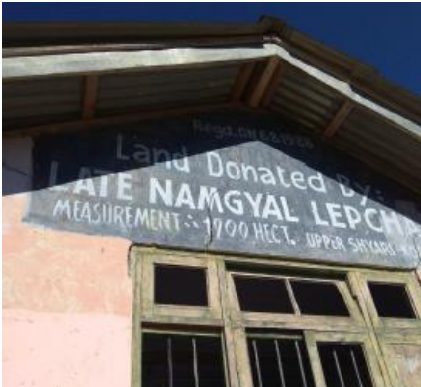
Picture 5.2 Risk Description: Cracks in the school building still not repaired
