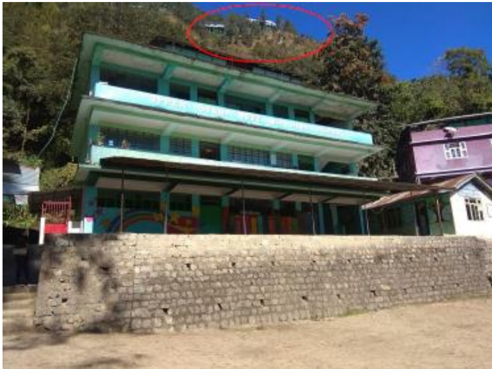
Picture 5.3 Risk Description: School building and the picture with red circle shows skywalk which has reduced the boulders fall at the backside.
