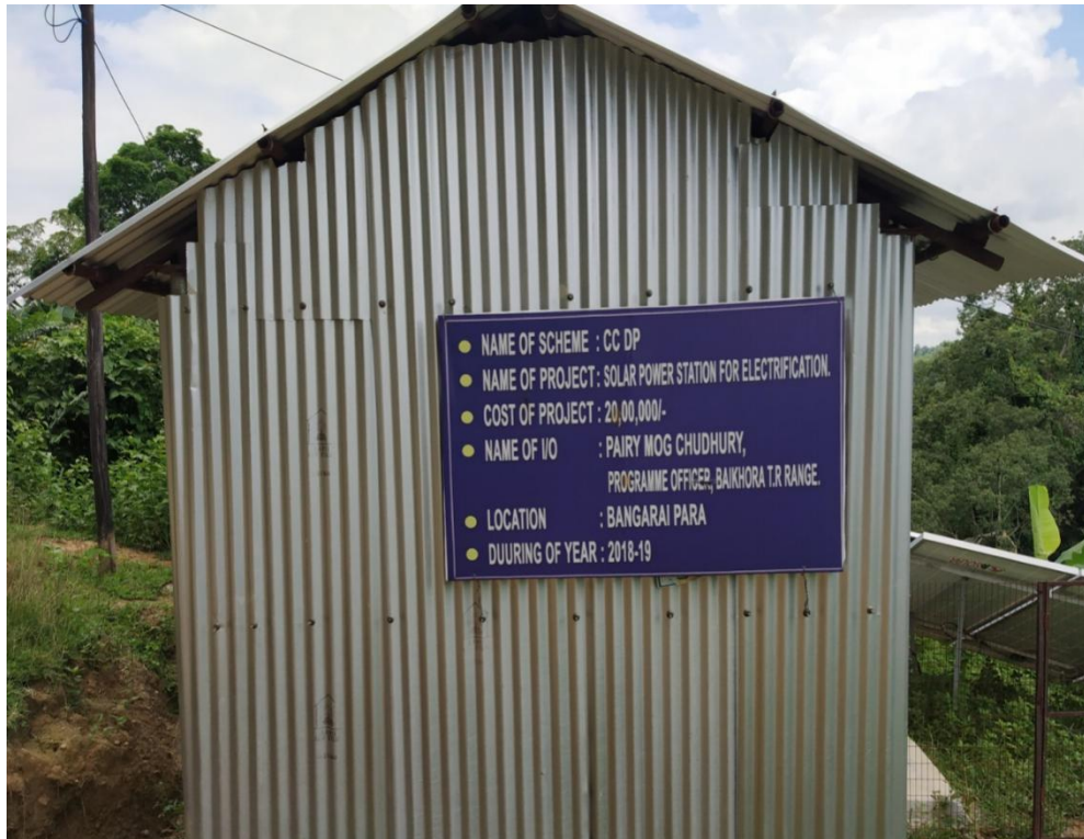
Solar Power House in Bangarai Para Village
