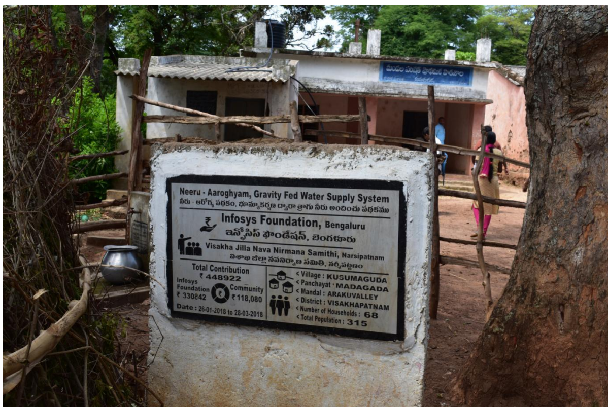
Gravity fed water supply system in Kusumuguda.
